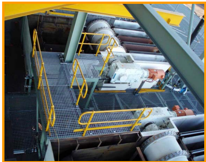
The two Boozer L4-Type disc filters in the filter building (without segments) – view from above to common access platform
