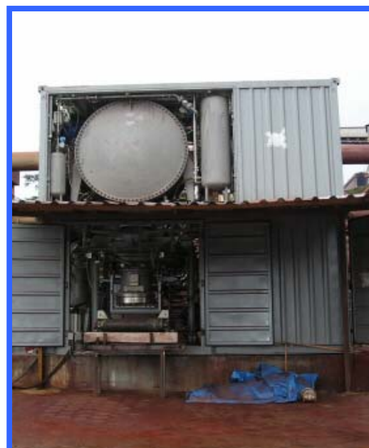
Test operation with the mobile pilot plant at the site in Brazil
