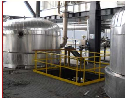
Two Hi-Bar Oyster Filters in a PTA plant
